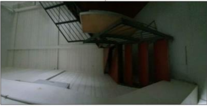
MAIN STAIRS (2 UNITS) INSTALL VINYL TILES IN REPAIR WORKING DESIGN AND TEXTURE AS APPROVED BY UP/CEBU/OCA. NOTE: FIX THE STAIR THREADS FIRST PRIOR TO INSTALLATION OF VINYL TILES.
